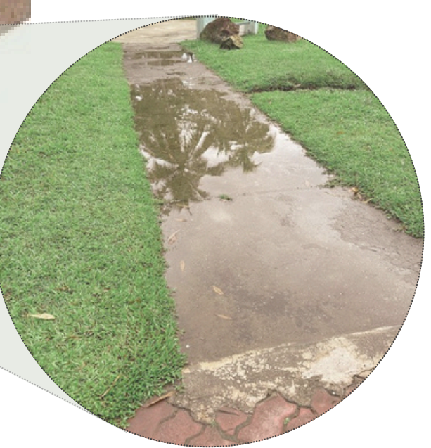
Water Pools form on Uneven Surfaces
